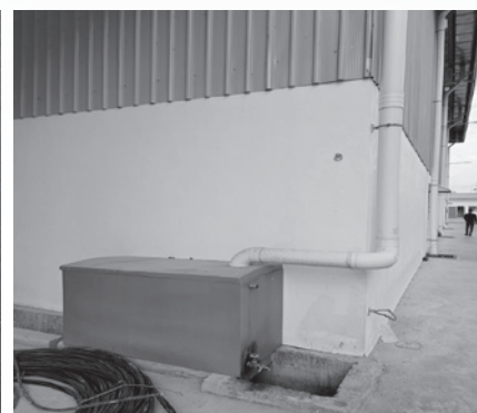
Rainwater harvesting tank
